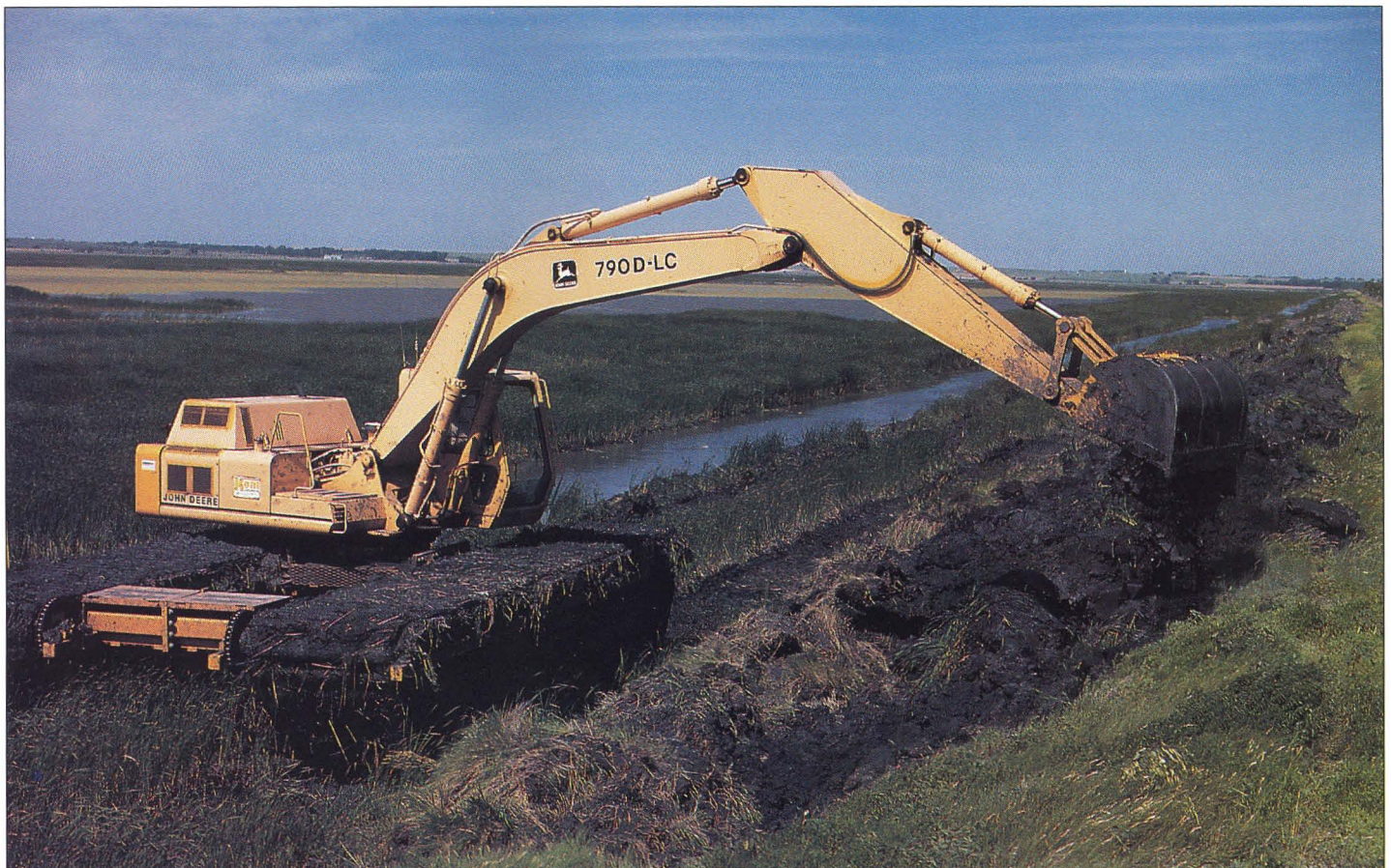
Goals of the Cheyenne Bottoms renovation are to handle the water received more efficiently so that even during drought years, some wetland habitat will be available. Construction will allow better movement of water between pools.
